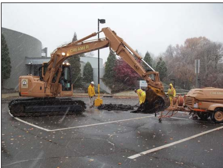
Employees of J. Fletcher Creamer & Son begin construction on the base and support system for the Huey helicopter at the NJ Vietnam Veteran's Memorial.
